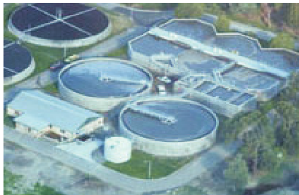
Fig. 8.7 (NCERT): Aerial view of a sewage treatment plant. The circular tanks are the aerator/settler combinations of the secondary treatment loop; the rectangular tank is the primary sedimentation basin.
