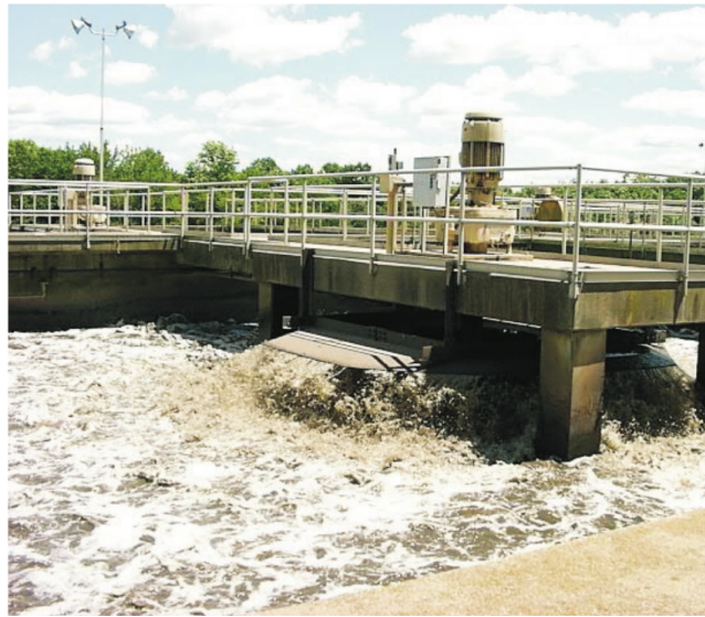
Fig. 8.6 (NCERT): Inside view of a secondary (biological) treatment tank — vigorous aeration is visible from the surface turbulence. Microbial flocs do the heavy lifting of digesting dissolved organic matter.
